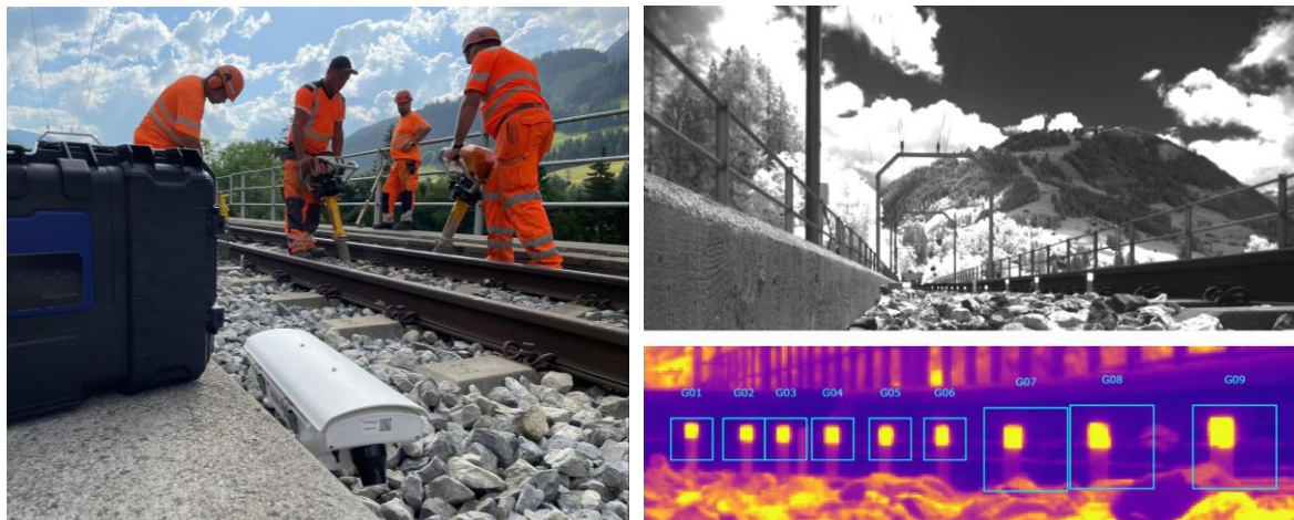
Left: Tamping operations monitored by the AIMsight system. Right: Detail of the optical tracking patterns on the rails.
